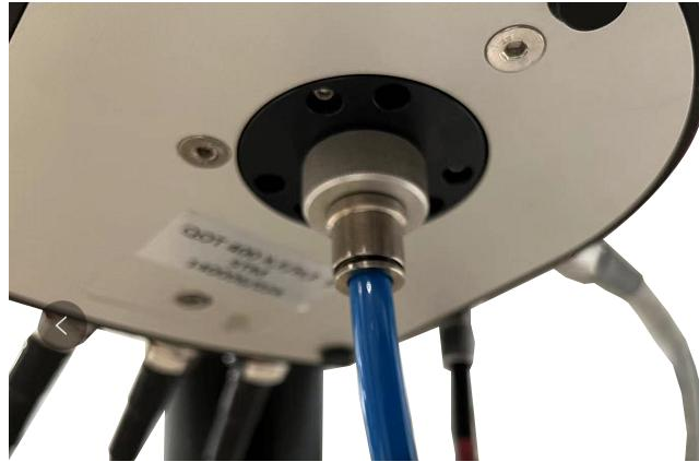
Figure 17. VT gas connection
