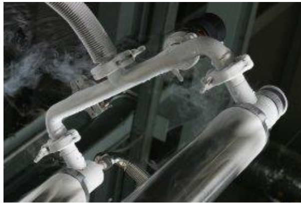
Figure 18 View from below the manifold showing water condensing in chilled air
