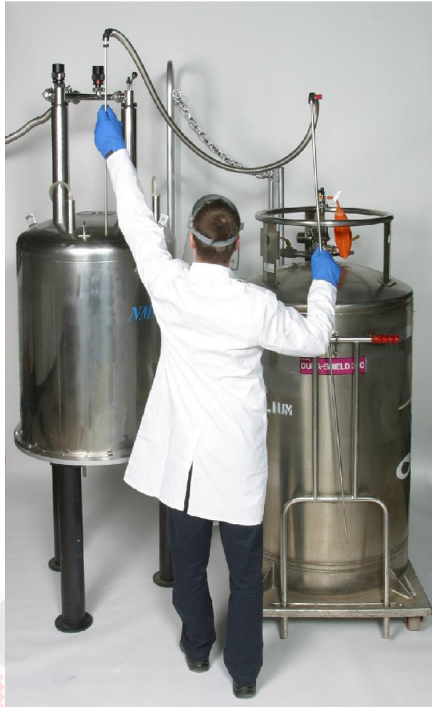
Figure 10 Siting of cryostat and storage dewar
