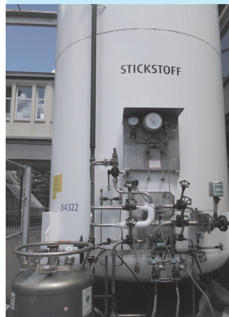
Fig. 4.2-1 Big liquid nitrogen tank of the Physics department, University Leipzig
